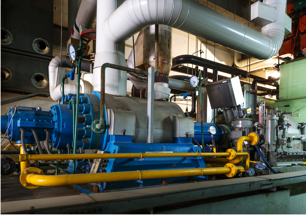
Figure 1. Modern gas fired boilers carry significant hidden costs including forced production down time, extensive maintenance requirements and emission permitting fees. Source: hxdyl/Adobe Stock
