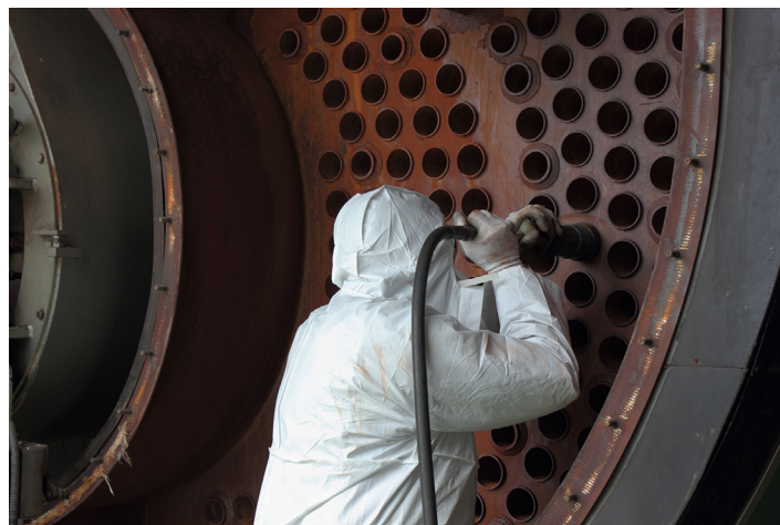
Figure 2. Routine maintenance procedures for a fossil fuel fired boiler include vacuuming and cleaning of radiant tubes. Source: markim/Adobe Stock
